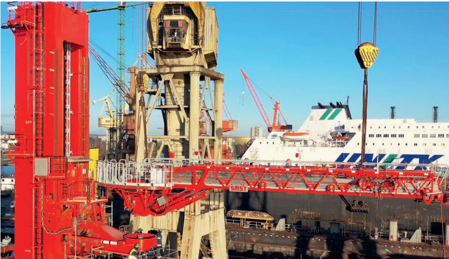
Once the tower had been installed, the next step was to mount a gangway
